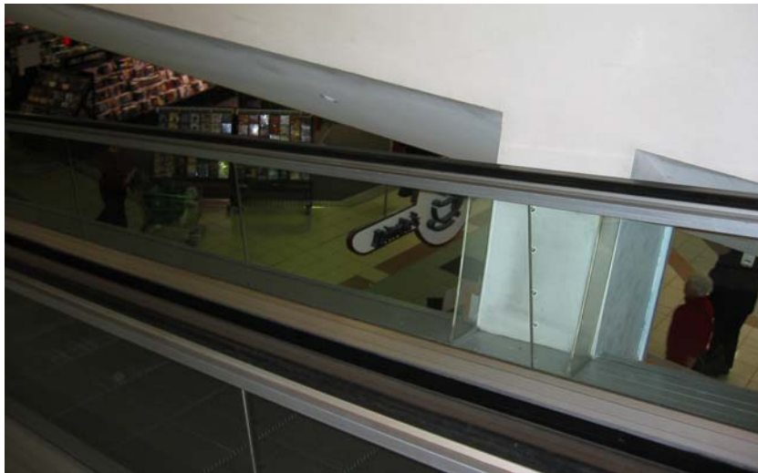
Trap points such as where escalators pass through floors have caused fatalities and should be guarded.
