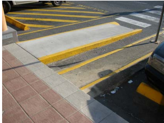
All potential trip hazards should be highlighted
