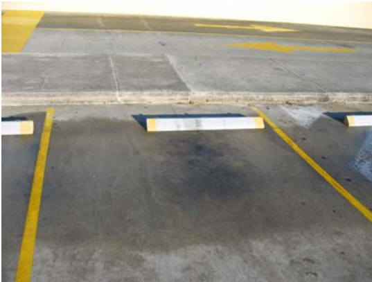
These shortened wheel stops still work effectively but reduce the trip hazard by widening the walking path,
